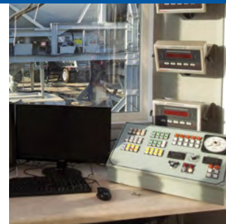
RC3 Batch Automation Controls
