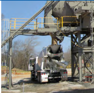
Mixer Maintenance Platform and Dump Cone
